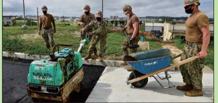
U.S. Navy Seabees deployed with Naval Mobile Construction Battalion (NMCB) 5, lay asphalt onboard Marine Corps Air Station Futenma, May 15.
