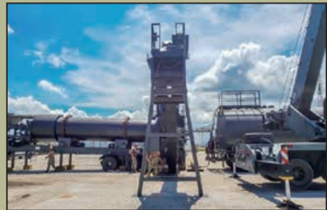
Seabees assigned to Naval Mobile Construction Battalion (NMCB) 4 conducts a mobile asphalt batch plant setup with NMCB 11 crane support, Aug. 21.
