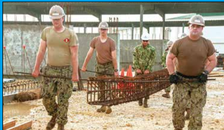
Seabees assigned to NMCB 3, move a rebar cage to a staging area during crane operations as part of a project to build a k-span structure onboard.
