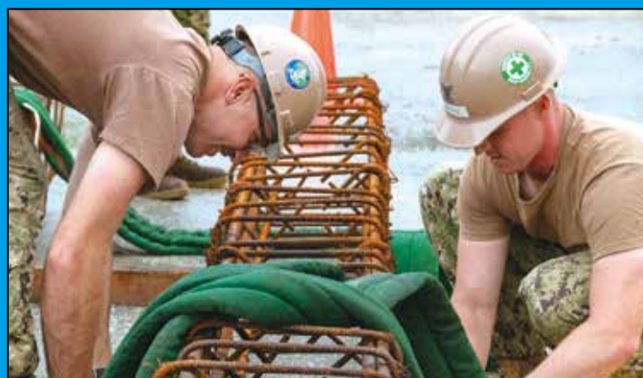
Seabees assigned to NMCB 3, position slings around a rebar cage during crane operations as part of a project to build a k-span structure onboard Camp Shields, Dec. 5.
