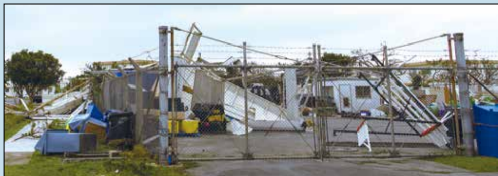
An 18th Force Support Squadron recreation center storage facility lies in shambles after Typhoon Trami, Sept. 30, at Kadena Air Base.
