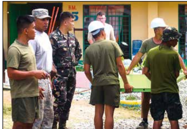
▲ Master Sgt. Juan AguilarMunoz, left, site 2 senior non-commissioned officer-in-charge with 18th Civil Engineering Squadron, observes door installation procedures on a 2-room classroom building during Exercise Balikatan at Alibagu Elementary School, Ilagan, Isabela, Philippines, May 3.
